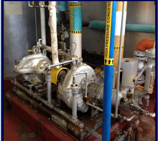
Inefficient Pumping System
