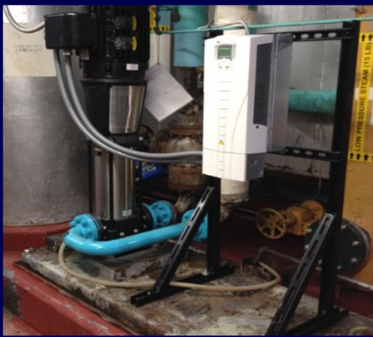
Newly Installed PS75 VFD & Pump
