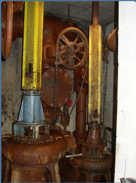
Leaking seals cause environmental hazard
