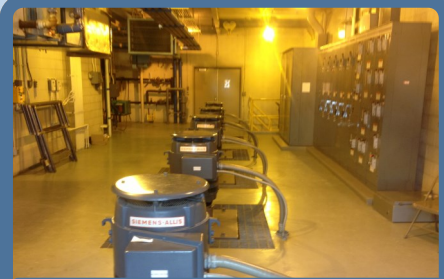
Bearing maintenance required
