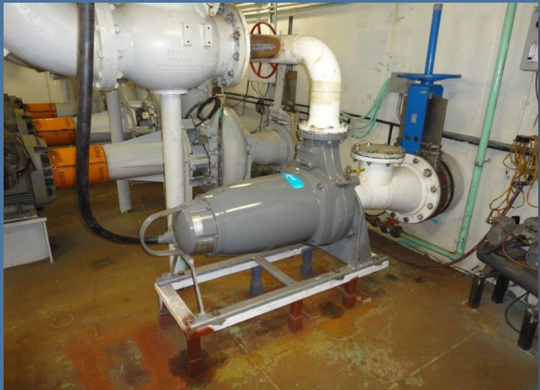
VALLEY PUMP STATION
