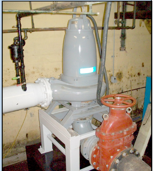
THE NEW FLYGT DRY PIT SUBMERSIBLE PUMP AND J&S GATE VALVE INSTALLED WITH NO PIPING MAZE AND NO SHAFTING
