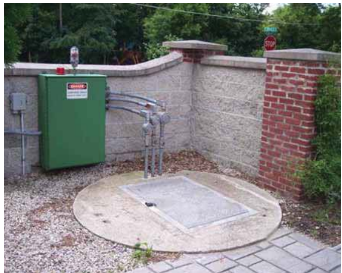
After a history of clogging problems, the Village of Hartland, Wis., first tested a new type of pump at its Crystal Drive Lift Station. The new equipment eliminated the clogging problem and unexpectedly used less energy.
