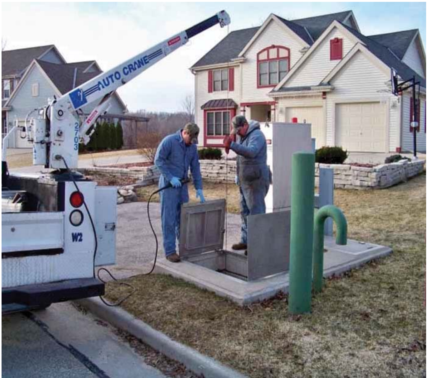
Jake Schlafer and Josh Georgenson, collection system maintenance operators with the Village of Hartland, Wis., make an emergency service call to service a clogged pump. Mike Gerszewski
