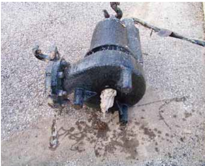
Clogged lift station pumps were common in Hartland until the village switched to a different type of pump. This pump’s inlet, where flow normally would enter, is plugged with disposable cleaning wipes.
