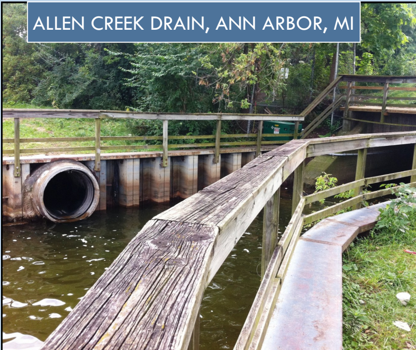
The 48" Tideflex CheckMate installed on the storm sewer at Allen Creek Drain, Ann Arbor, MI.
